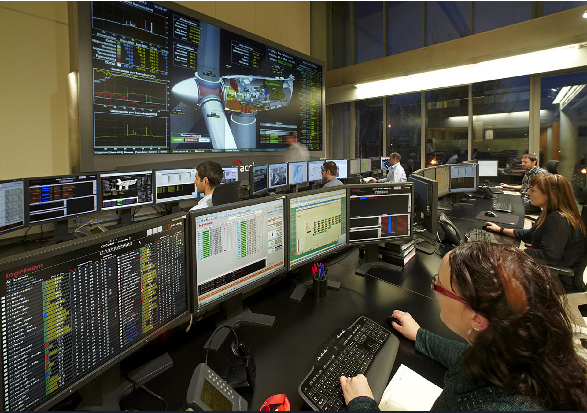
CECOER. ACCIONA Energy renewable facilities control center
