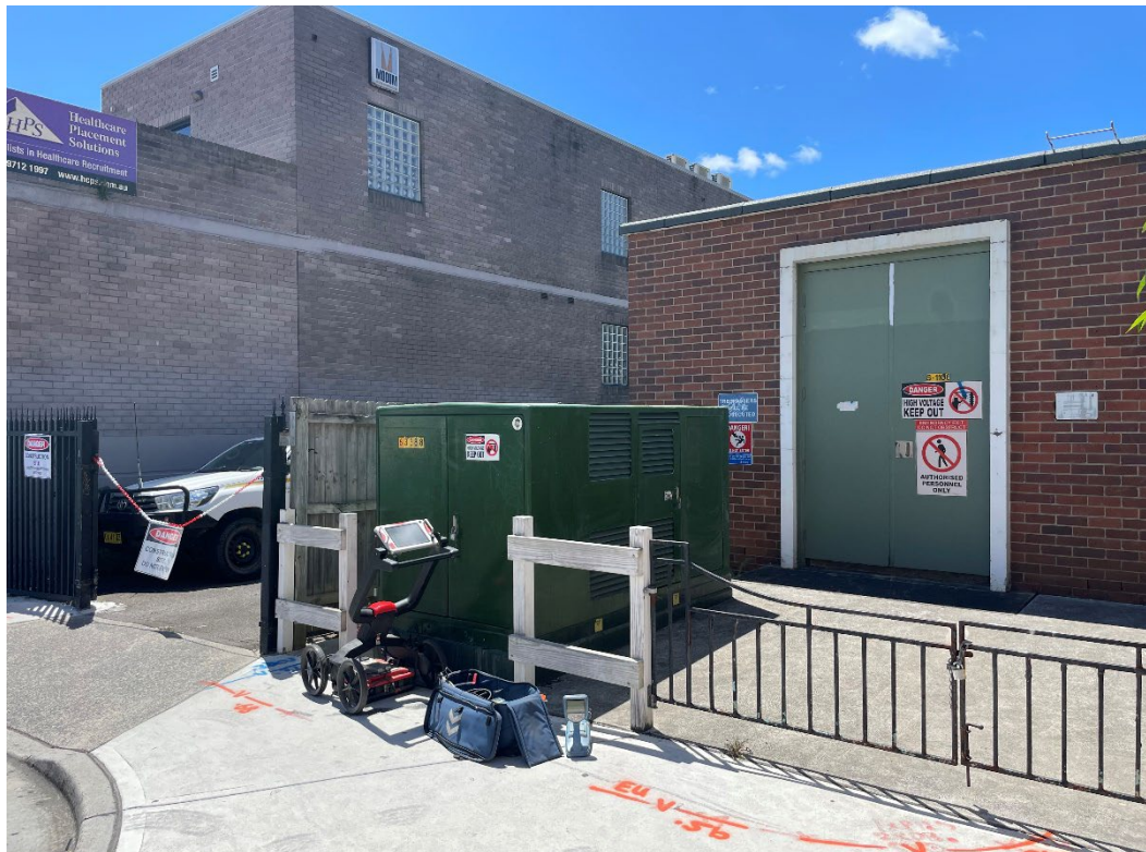
Plate P5: Electrical substation south of the western construction zone (facing northeast)
