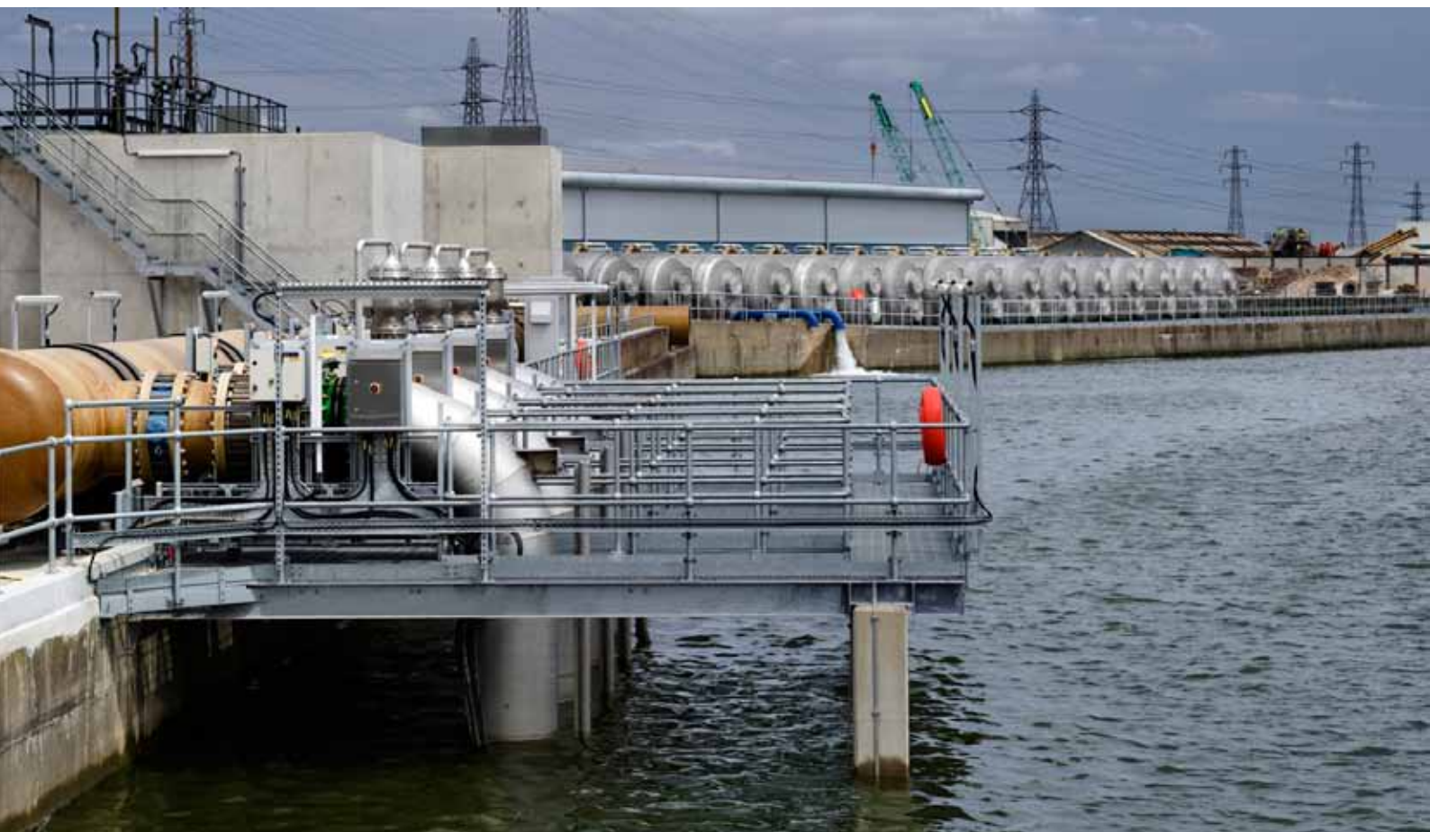
Beckton desalination plant. London, UK.
